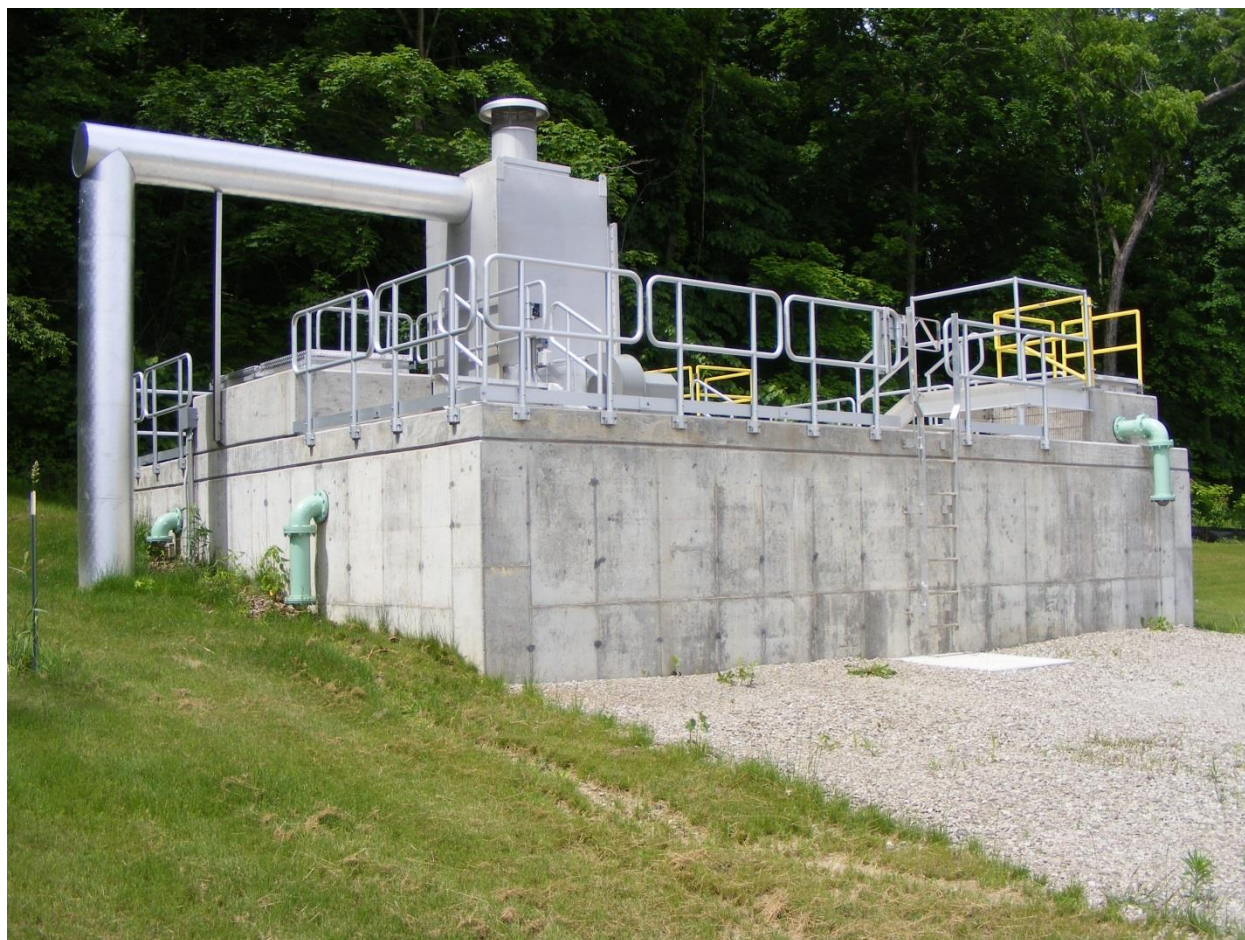
Aeration followed by Detention Tank
