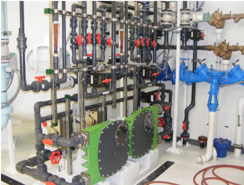
Chemical Feed and Backflow Prevention
