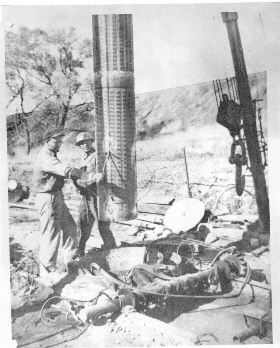
Placing screen in well showing centering guides on screen to assure proper placement of screen.
