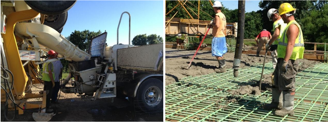
Figure 8. Concrete being discharged to a pump truck and then to the deck
