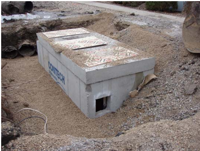
Grit Collection Chamber (Site H8)
