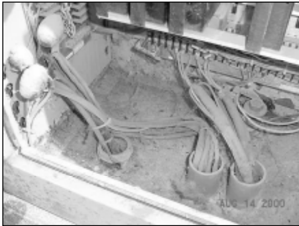
Figure 13 Dirty Cabinet at Intersection 20
