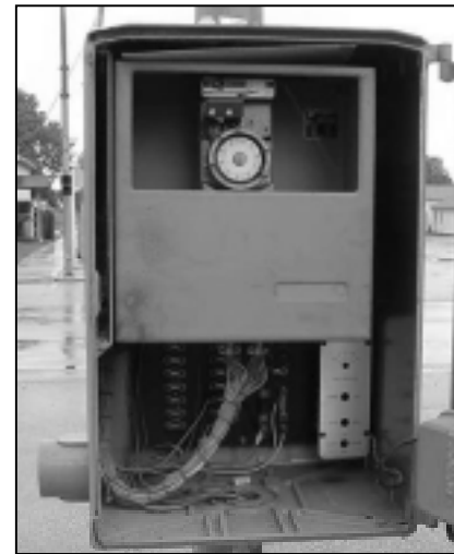
Figure 6 Controller Cabinet at Intersection 06
