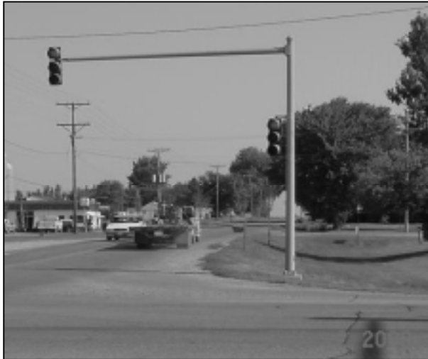
Figure 11 Missing Backplates at Intersection 17
