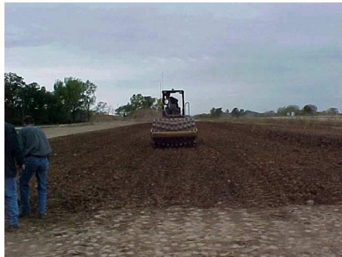
Figure 11. Compaction being performed by CAT CP-533E roller in reverse direction for test strip 2A
