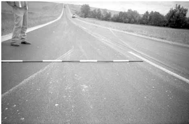
Rutting in the newly-placed first lift.
