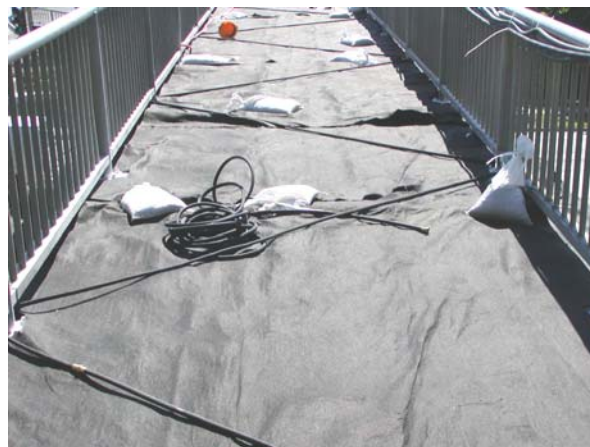
Figure 12 ECE System in Place
