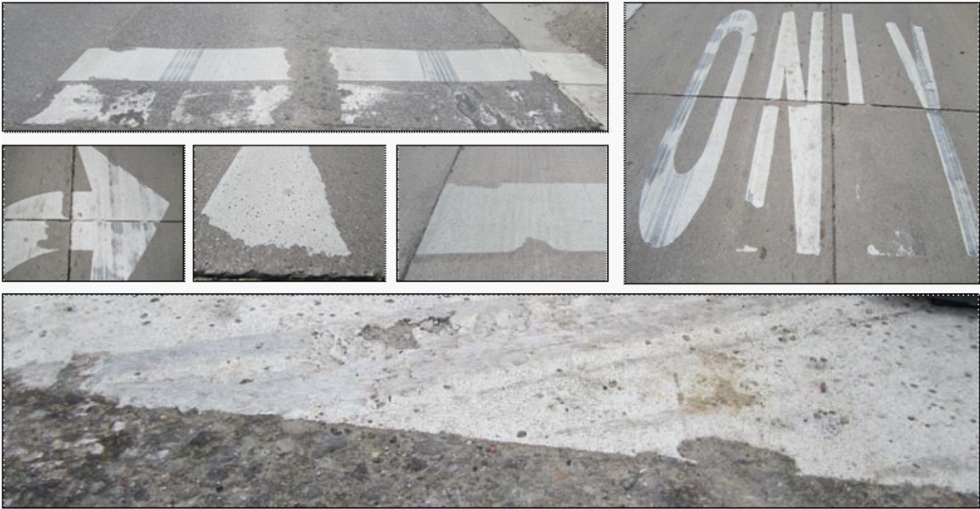
Transverse marking wear and snow plow damage
