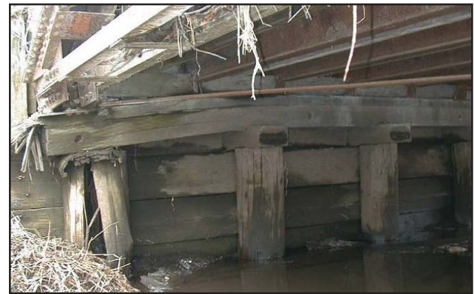
Biological deterioration resulting in reduction in pile cross section (top) and complete deterioration of a pile section causing failure of pile cap (bottom)
