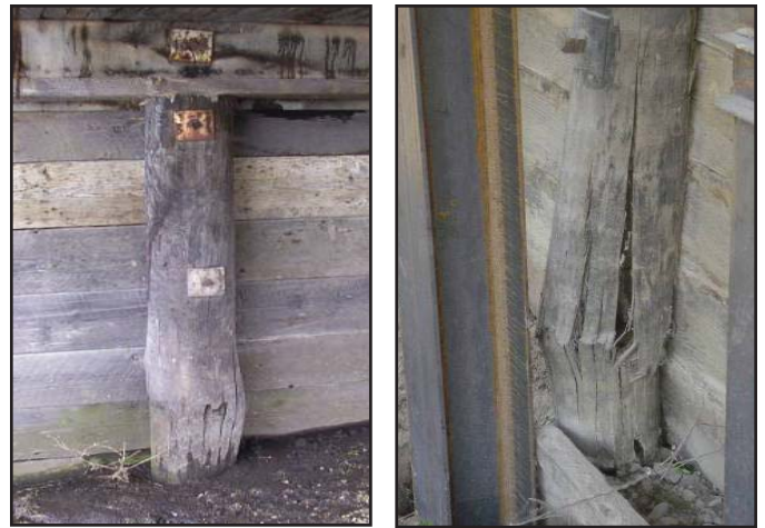
Compression failure of deteriorated pile section caused by overloading leading to bulging of timber fibers (left) and mushrooming of the pile section (right)
