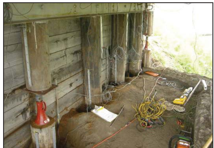
Pile sections removed to simulate timber pile deterioration
