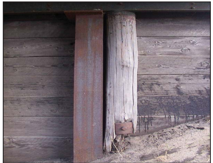
Steel pile driven adjacent to a defective timber pile
