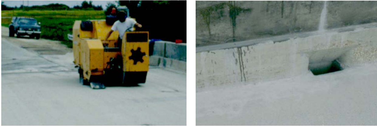
Photographs showing Turbo Blast shot blasting machine (left), and grinding of curb and gutter (right).
