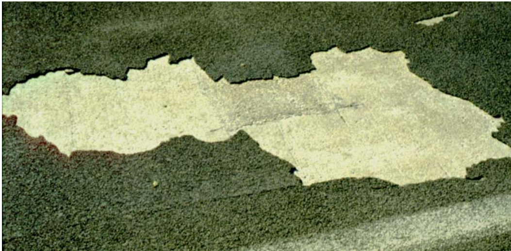
Photographs showing delamination of Flexogrid.
