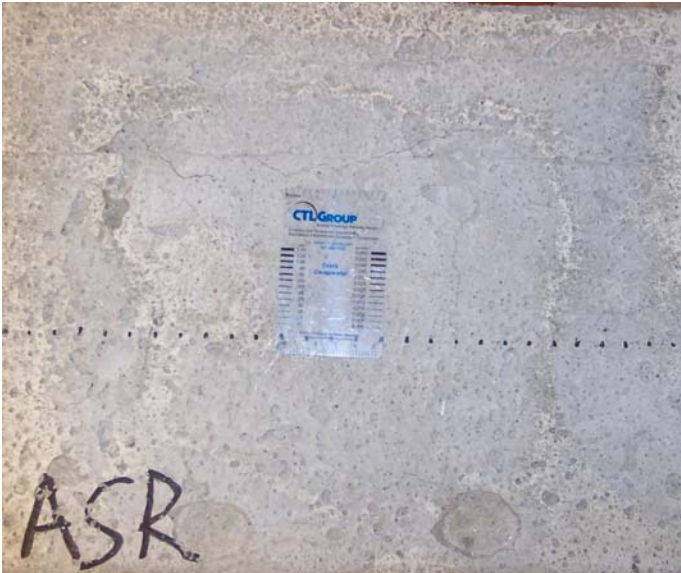
Figure 8. Surface cracking on the specimen containing ASR-reactive aggregate
