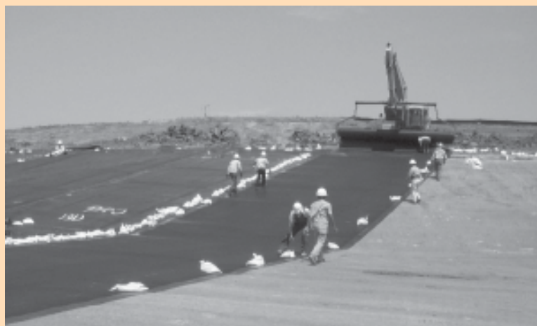
Workers install the new Subtitle D liner in the Phase 1B area of the Metro Park East landfill.
