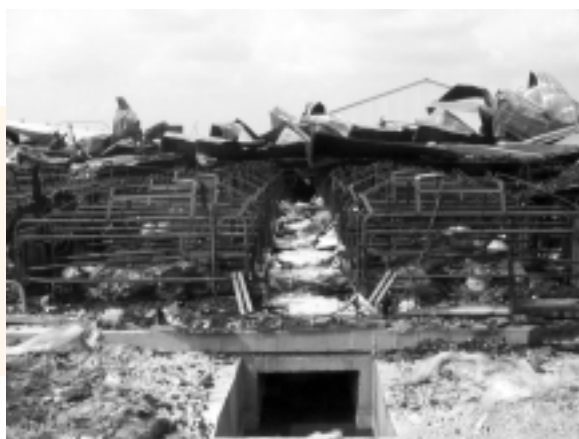
The remains of a swine confinement facility after a fire.
