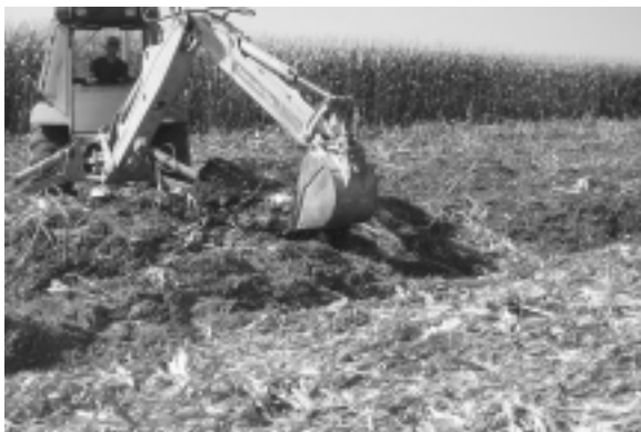
Beginning construction of a composting windrow after a fire at a sow facility.
