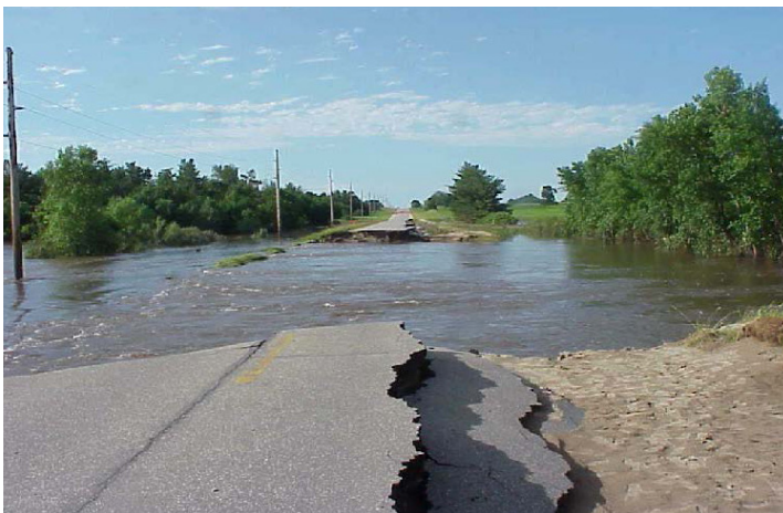
IA 150 near Vinton during 2008 flooding (Image: ©Iowa Department of Transportation)
