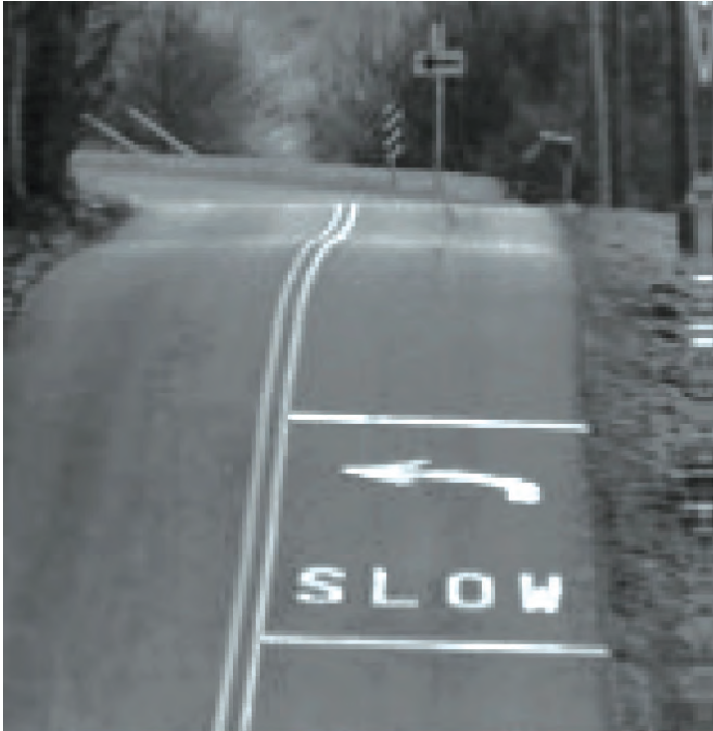
Figure 6.19. Test site pavement markings (Retting and Farmer 1998)
