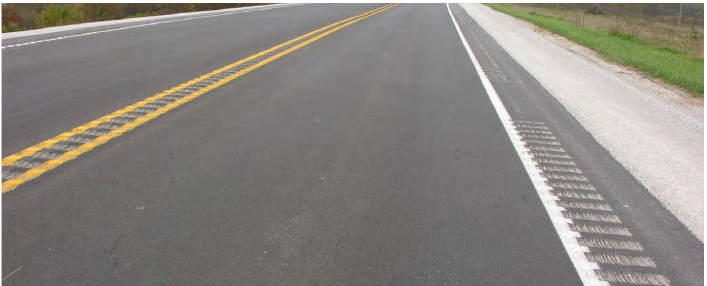
Figure 3.13 Gapped milled-in shoulder rumble stripes on US Highway 34 near Creston, Iowa (Roche 2011)
