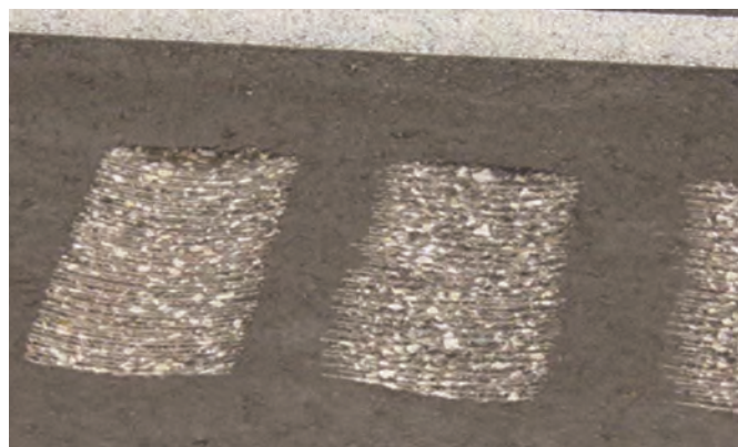
Figure 3.7. Milled shoulder rumble strips (Iowa DOT)
