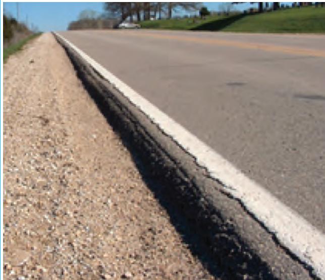
Typical rounded edge on asphalt
