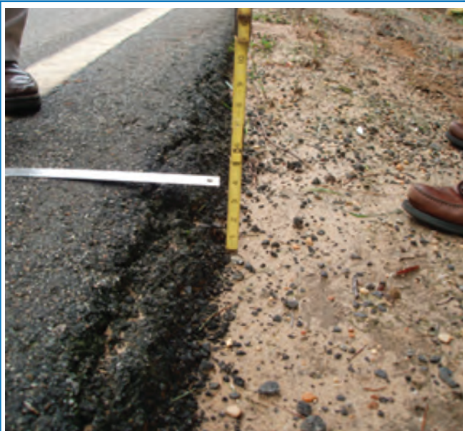
Pavement edge after resurfacing without Safety Edge
