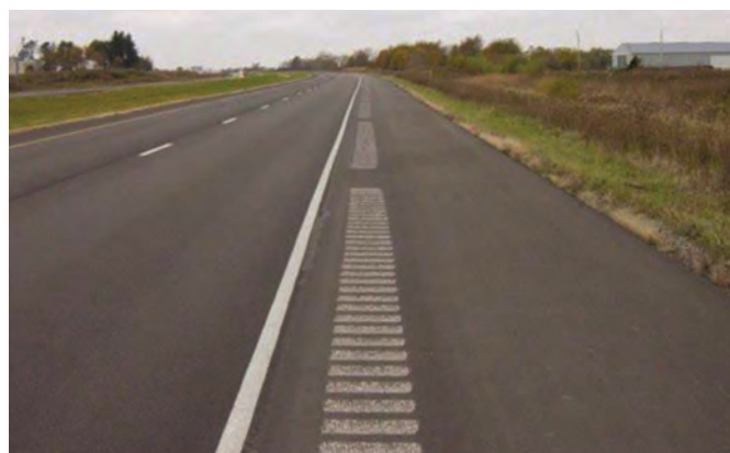
Figure 3.8. Gapped shoulder rumble strip pattern provides bicyclists with crossover spaces (Iowa DOT)
