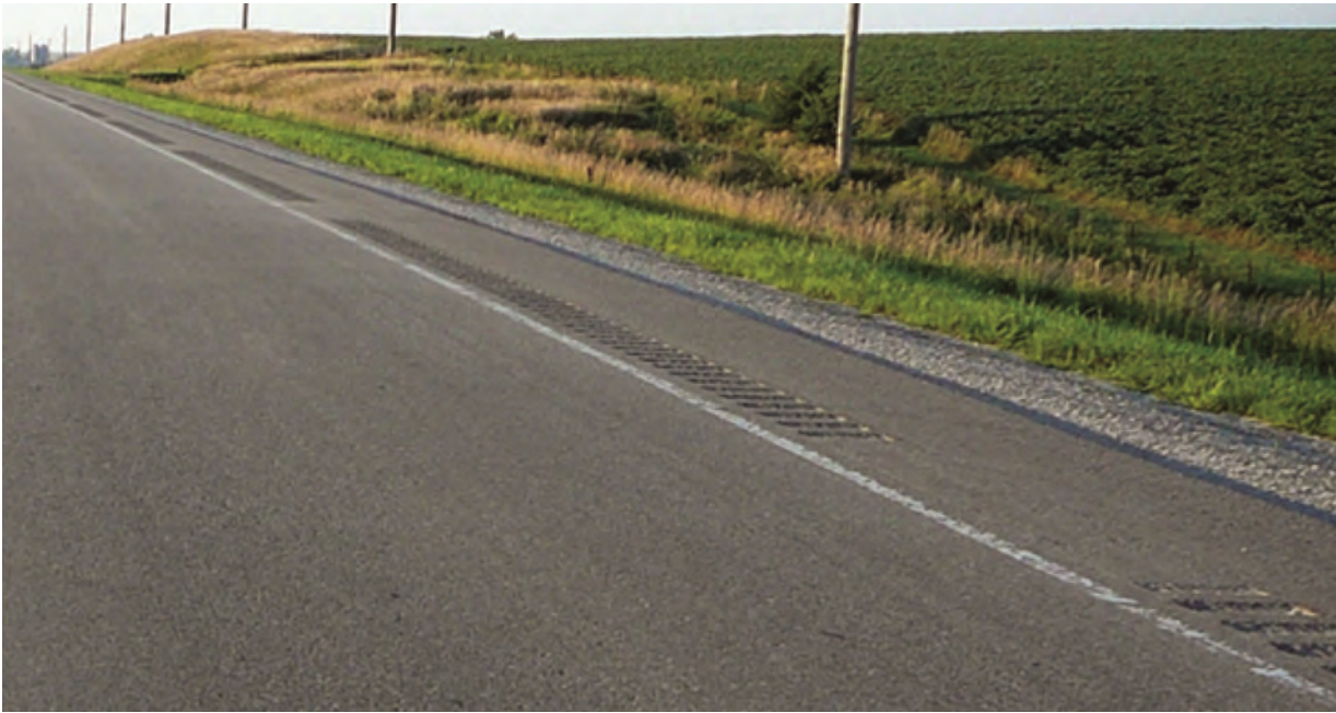
Figure 3.9. Gapped milled-in rumble strips on a state highway with 4 foot paved shoulders
