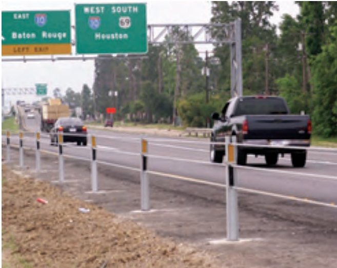
Figure 5.4. Trinity Highway Products Cable Safety System (CASS™) (Alberson 2006)
