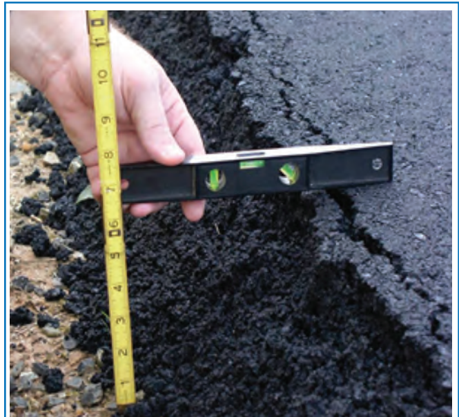
Pavement edge after resurfacing without Safety Edge
