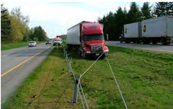
Figure 5.2. Prevented cross-median crash by a cable median barrier (Washington State DOT)
