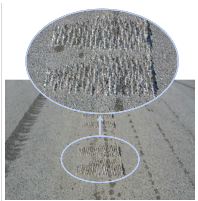
Figure 4.3. Uneven CLRS milling (Michigan DOT 2009)
