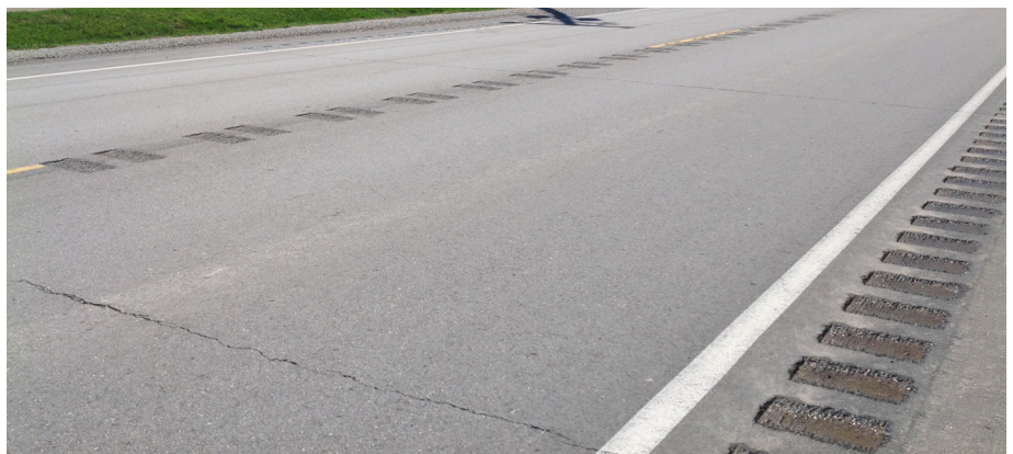
Reflective cracks in non-interlayer overlay on US 169 in April 2014
