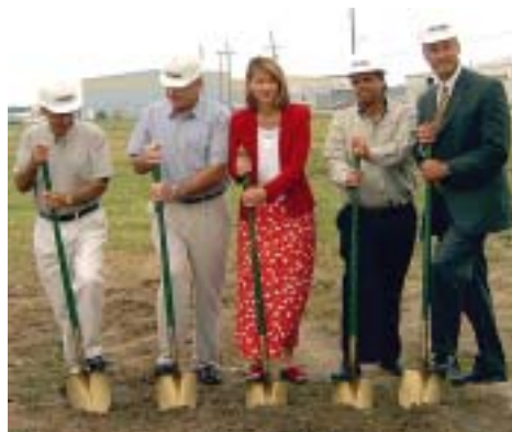
Breaking ground for the snow removal equipment storage building at Sioux Gateway.
