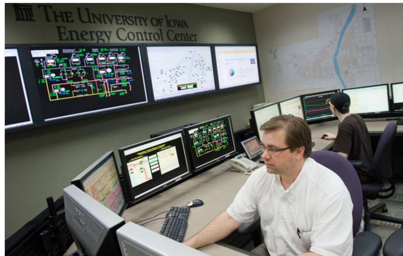
With the new Energy Control Center, Facilities Management staff members, such as George Paterson (foreground), now have power at their fingertips—not only to manage campus energy resources from a central location, but also to reduce the University's carbon footprint by streamlining energy usage.
