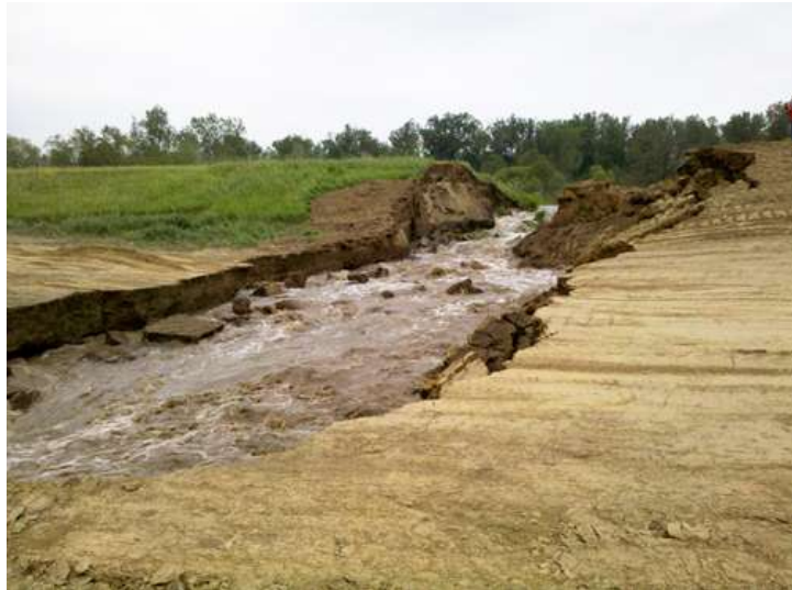
Figure 2: Levee Failure in Hamburg, Iowa (Source: Iowa Department of Public Safety)
