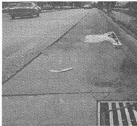
Fig. 1 Cold mix was used to reduce the dropoff after adjacent pavement slabs settled along a longitudinal joint.
