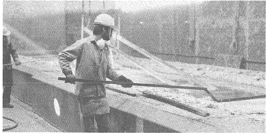
In the galvanizing process, the guard rail components are cleaned, fluxed, and placed in a kettle of molten zinc. This kettle holds 1.3 million pounds of zinc.
