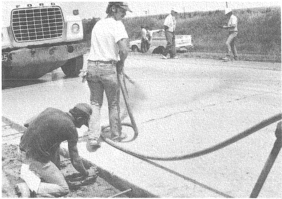
Dowel bars spaced about 2 feet apart and anchored into the edge of existing pavement with a 2-component epoxy are being cleaned just ahead of the paver. The surface of the existing pavement is being treated with a water-cement grout to serve as a bonding agent between the old concrete and the new overlay.
