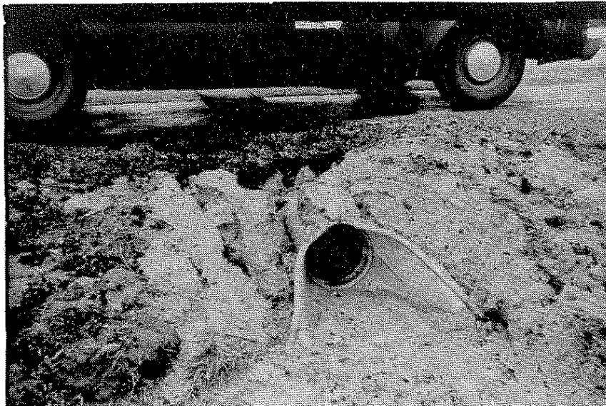
Figure 11: Erosion Around the RF-22 Outlet
