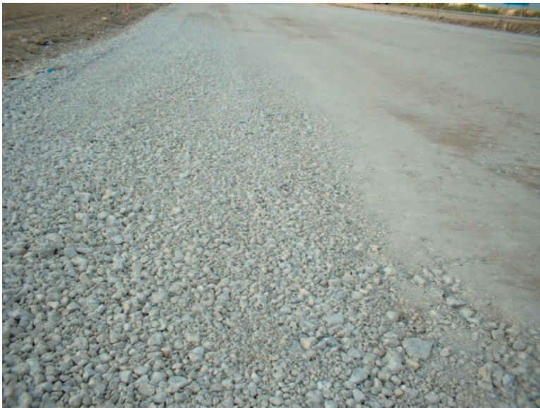
Segregation of fines in final base layer
