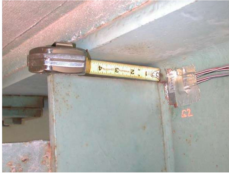
Figure 3.7. Typical web gap in negative moment region.
