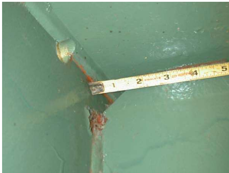
Figure 2.7. Photograph of typical web gap.
