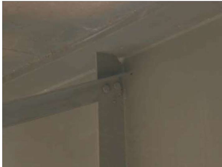
Figure 4.6. Photograph of typical web gap.
