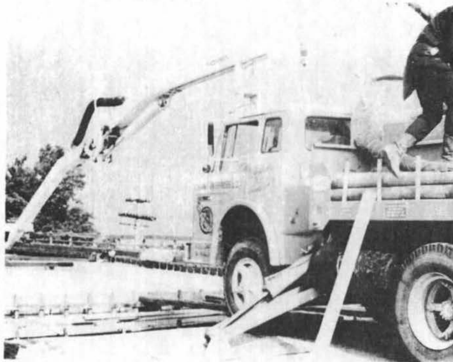
8 inch double piston pump with 5 inch discharge hose to the bridge floor.
