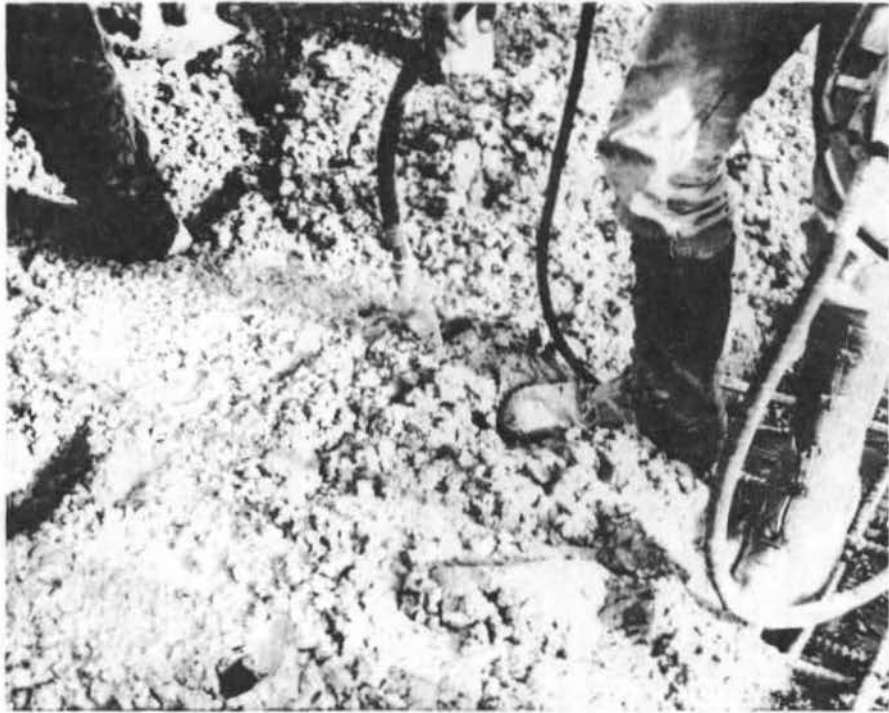
Vibrator not too effective after 40 to 50 minutes from batching - note hole left by vibrator in lower left of picture.
