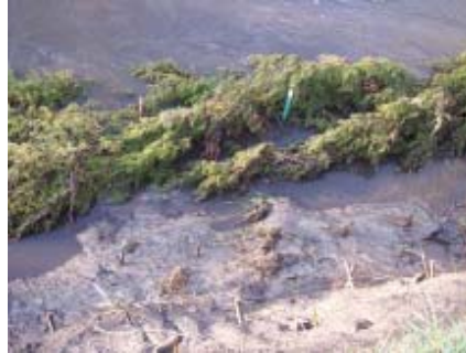
Figure 2. Looking across the revetment (bottom of the photo is the bank, top of the photo is the middle of the stream). Over two feet of sediment was deposited from an April 26, 2009 rain storm. Photo was taken on April 28. Note the two T-posts used to secure the base and top of each cedar tree and the willow cuttings just sticking out just above the sediment.
