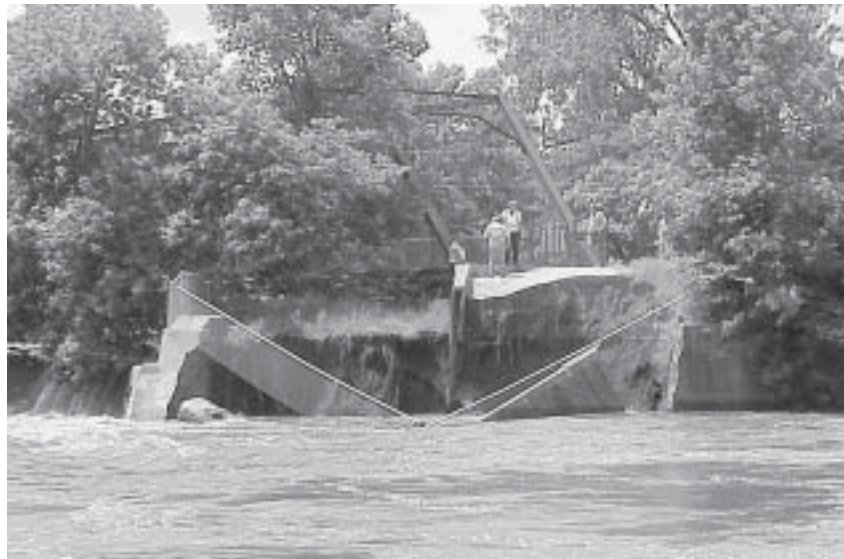
Surveying the damage at the Adel dam on the Raccoon River
