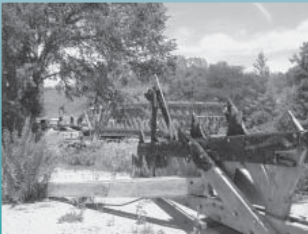
Reconstruction of the Cedar Bridge in Madison County is continuing and expected to finish in time for a dedication ceremony in October.
