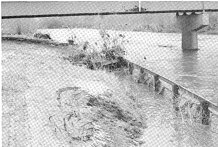
Figure 48. U.S. Highway 34 Bridge over East Nishnabotna River, Viewed Downstream from Left Bank of River
