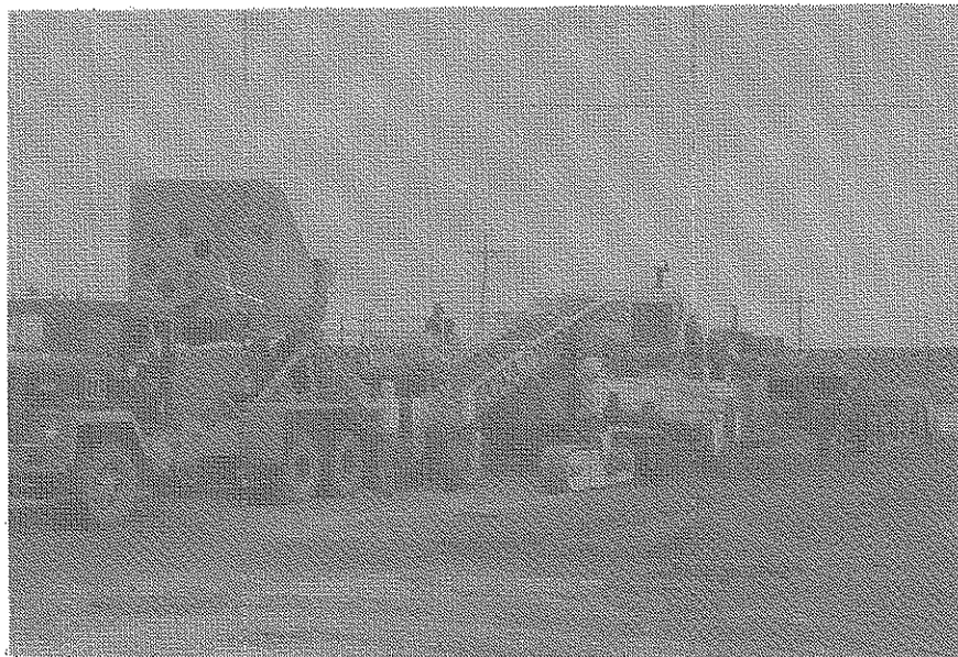
Mix was dumped onto the belt of the subgrader and placed ahead of the paver
