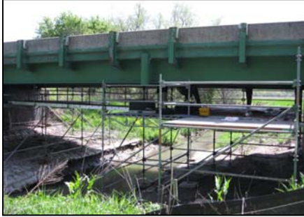
Figure 5 Scaffolding used to access the superstructure of the field bridge using operational/traffic loads as excitation
