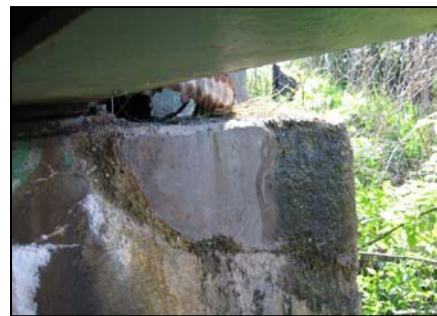
Figure 10 Photo showing actual cracking correlated with motion of exterior beams at 13.5 Hz
