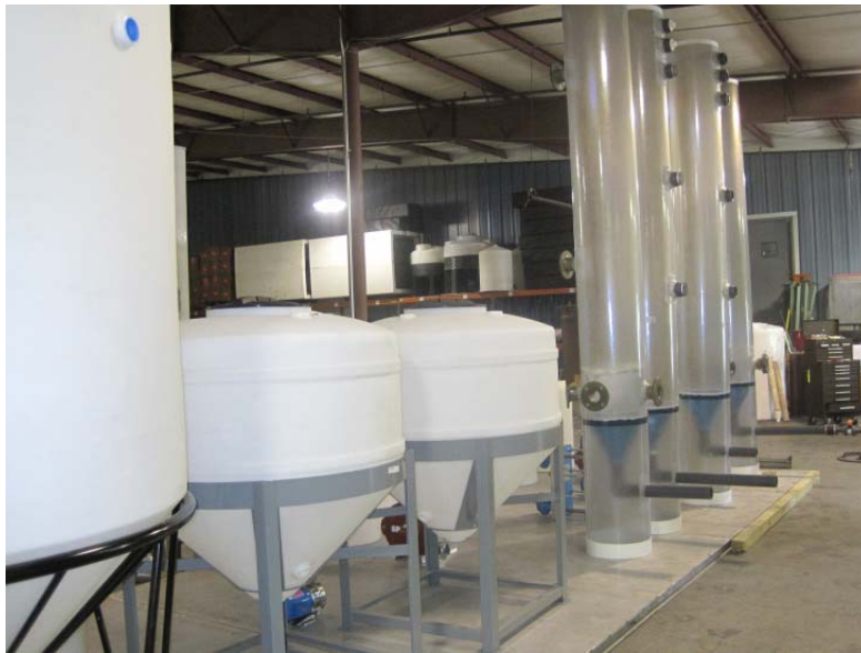
Pic # 3 Shenandoah pilot skid unit (front view)
