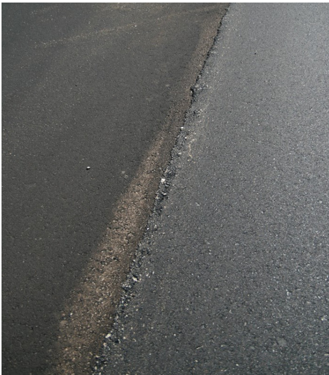
Longitudinal joint with fine segregation
