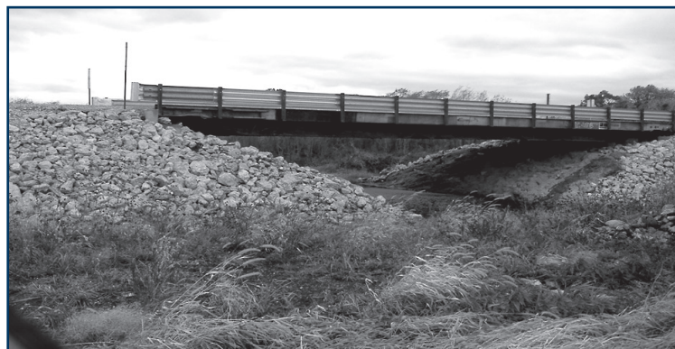
Completed Hoods Bridge, Buchanan County (Note the concrete-covered riprap under the bridge)
