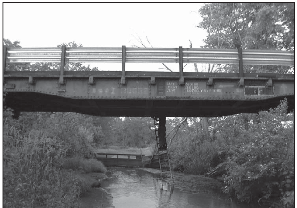
With careful design, engineering, and analysis, Buchanan County is experiencing success with cost-effective railroad flatcar bridges.
