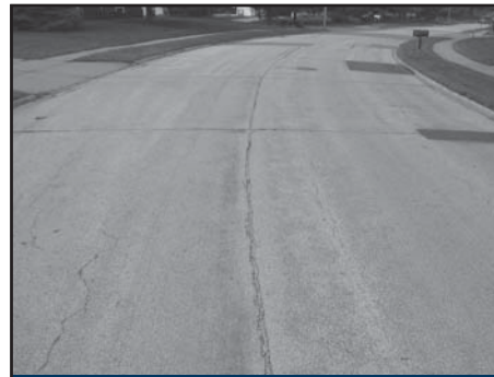
Figure 5. Reflection cracking. Photo courtesy of CCEE Department, ISU.
