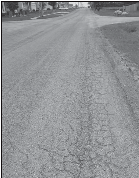
Figure 2. Fatigue cracking. Photo courtesy of CCEE Department, ISU.
