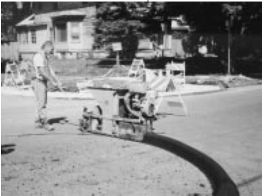
This temporary asphalt curb was installed during the summer of 1998. It has since been replaced with a permanent concrete curb.
