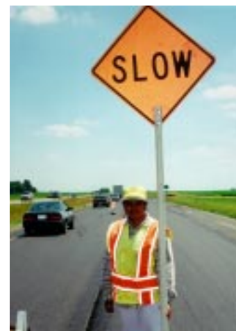
A flagger in the I-35 work zone sports the new safety vest and hat the Iowa DOT is experimenting with this year.
