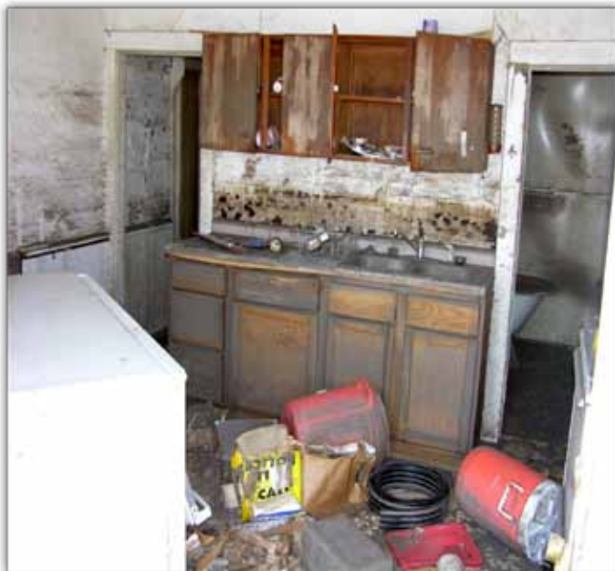
Figure 8. A Cedar Rapids home damaged by the 2008 flood.
