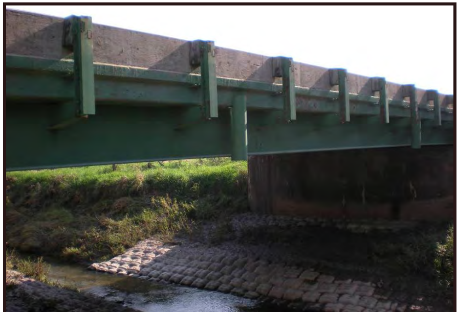
On-the Spot damage detection field testing on County IA-1, South of Iowa City, Iowa, near Gingerich Road
