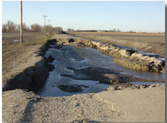
Photo taken in late November shows damaged roadway near Hamburg in Fremont County.
