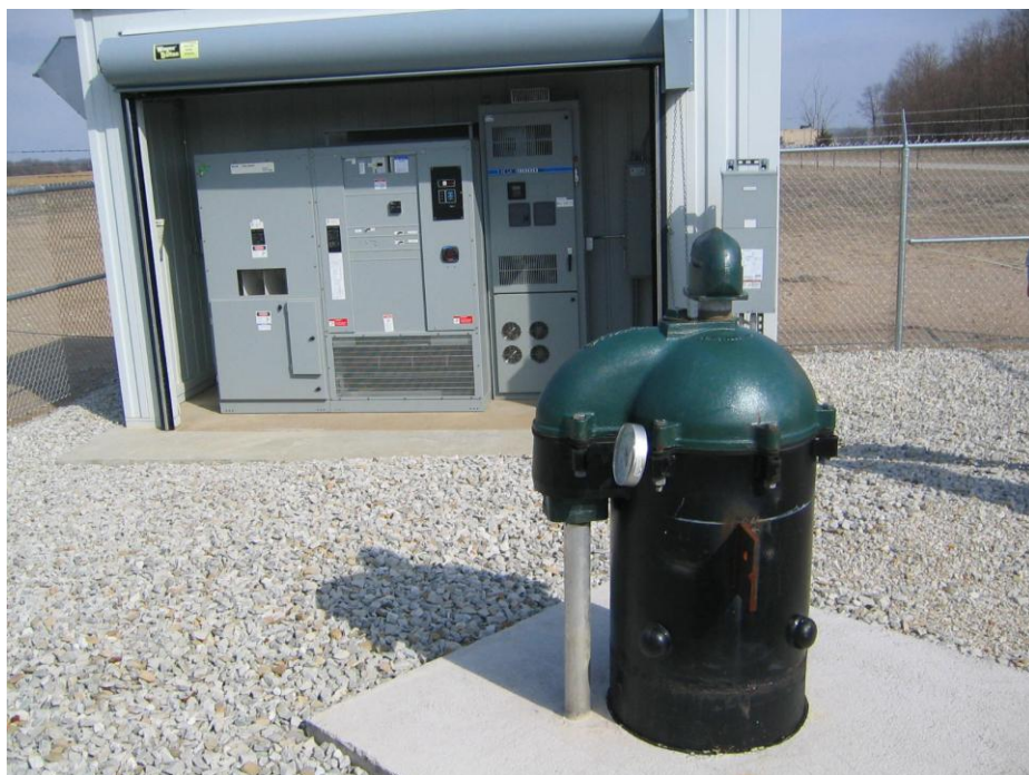
New well and controls installed as part of a DWSRF project completed in 2011
