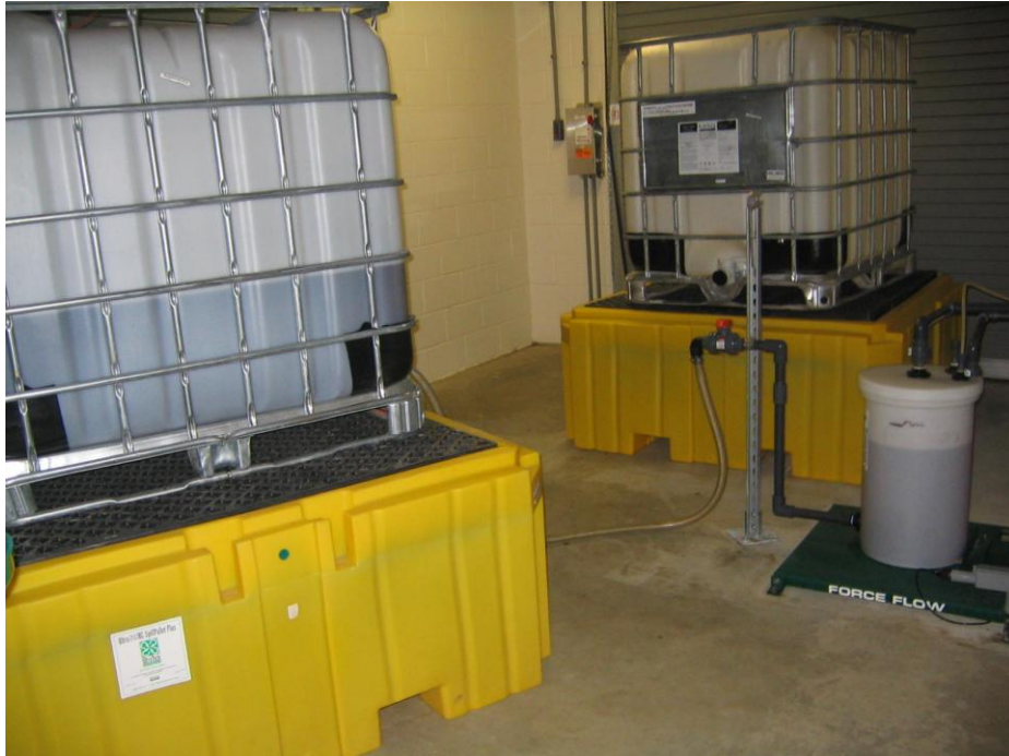
Chemical totes above containment tubs and day tank on scale, installed as part of a DWSRF project completed in 2011
