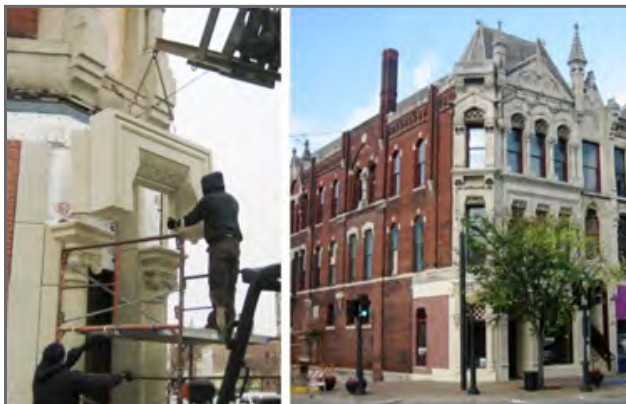
Installing the recreated limestone storefront at the Hedge Building. (Photos: Steve Frevert)
