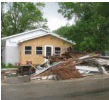
Flood-damaged homes, like this one in Oakville, are still being gutted and rebuilt.
