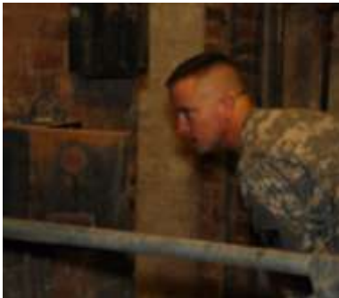
Col. Shawn McGinley, USACE, examines flood damage in the Veteran's Memorial building in Cedar Rapids.
