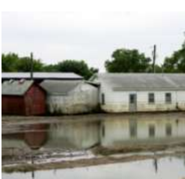
Buildings displaced due to the flood pile against one another in Oakville.
