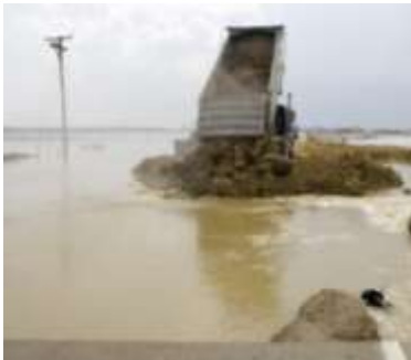
A truck dumps a load of rock into a levee breach in Oakville.
