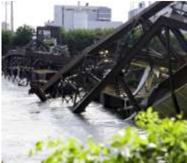
Gravel-filled railcars were not able to keep this Cedar Rapids bridge from being pulled off its pilings.
