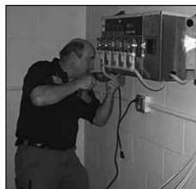
IPI Sales / Service Representative Kevin Peterson installs laundry equipment at the Iowa Medical & Classification Center.
