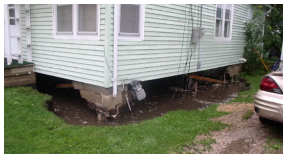
Damage sustained by the foundation of a home in Oelwein. Photo courtesy Randy Frank, Fayette County Emergency Management.
