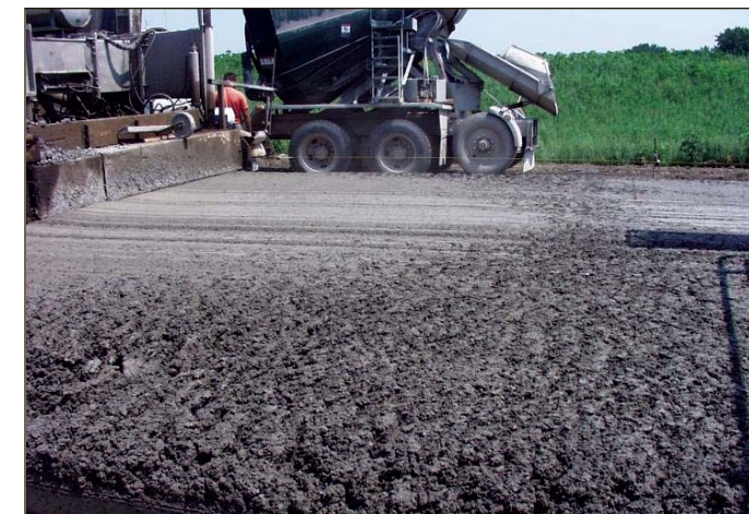
Figure 2. Segregated concrete (photo by Iowa Department of Transportation)
