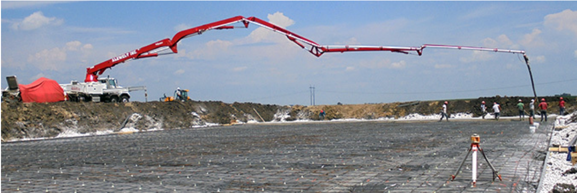
Spring construction – Get your rebar in a row, and follow concrete tips for an enduring structure.
