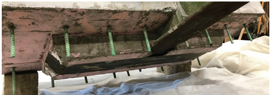
Completed integral diaphragm of the joint specimen before aggregate finish exposed under the form retarder, completion of the connection, and pouring of the UHPC into the joint
